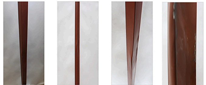
Fig. 5. Damaged steel frame images.
